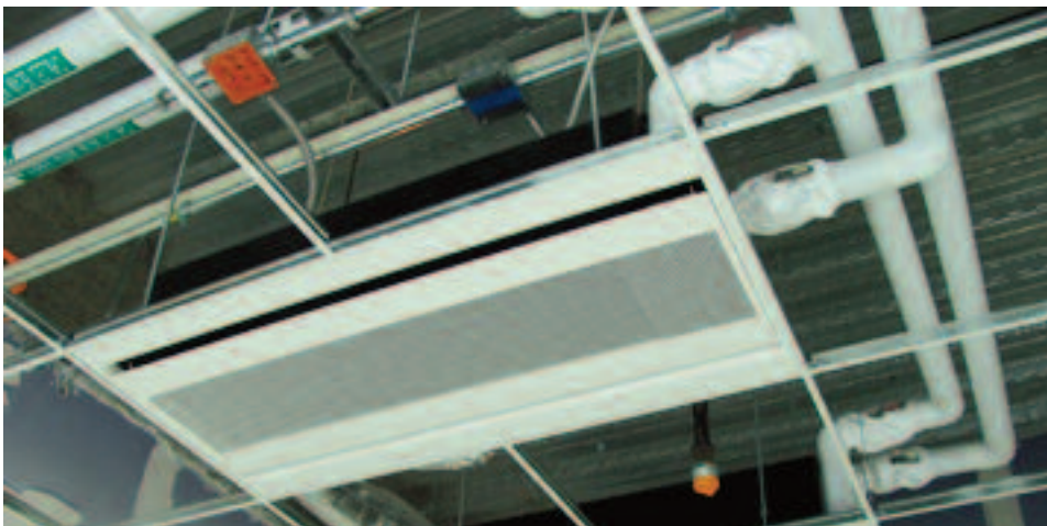
Active chilled beams installed for office application
